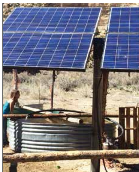
A solar pump water well.
